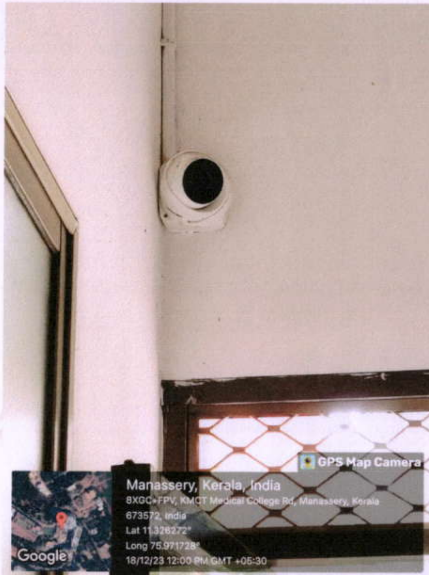
CCTV camera installation
